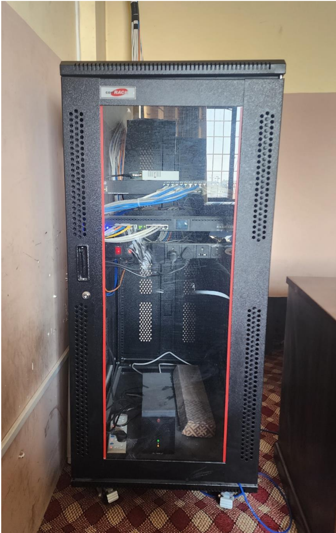
Annex 172, Photo of Central Networking System
